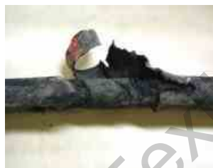
Fig: 15.23 Over heating of a cable
