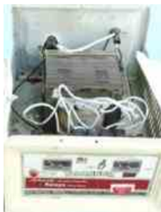
Fig: 16.20 Transformer in stabilizer
